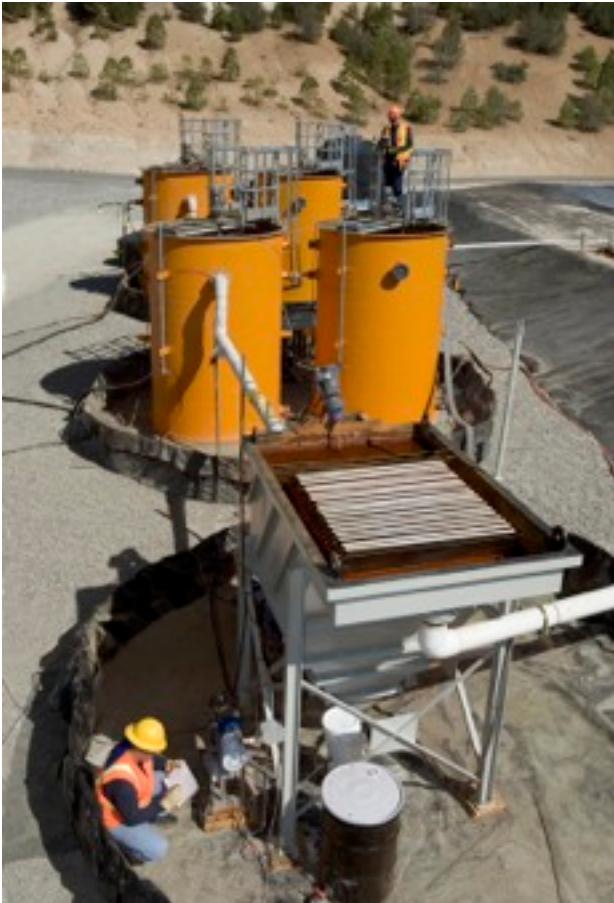
60 gpm high density sludge pilot system
