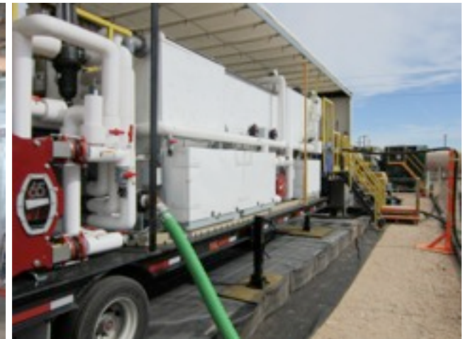
40 gpm trailer-mounted pilot system
